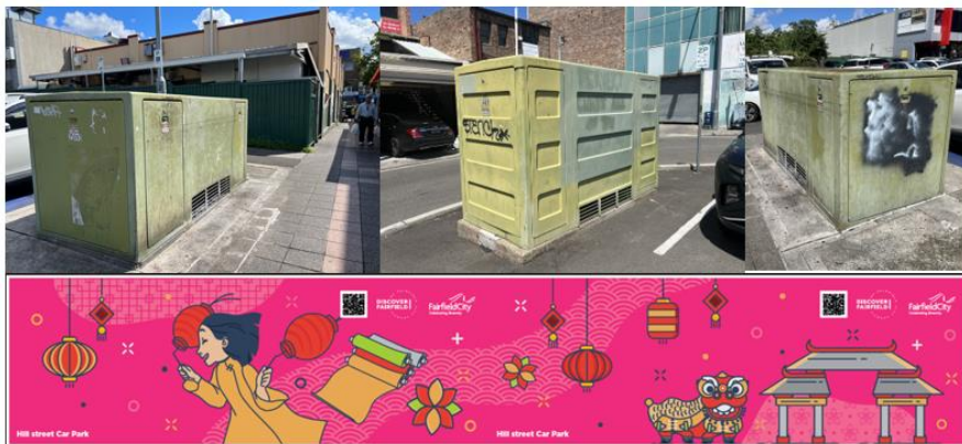
Proposed decal on 5 Endeavour Energy utility boxes in Cabramatta Town Centre.
