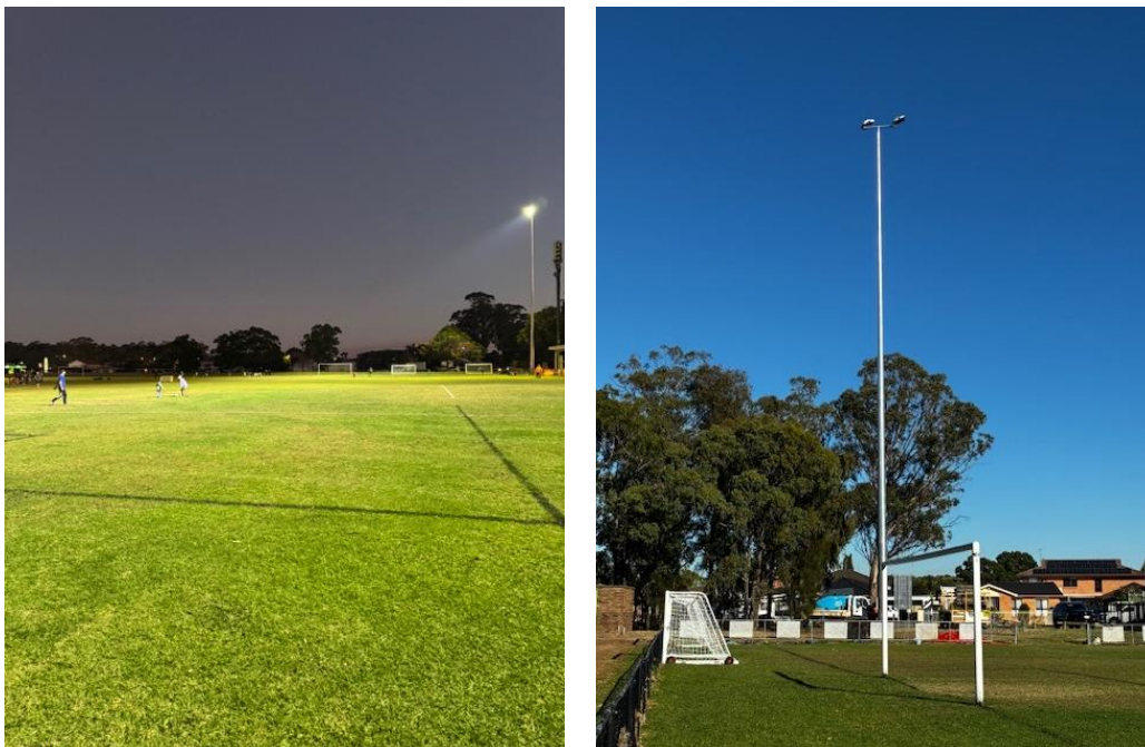
Figure 1 Stage 1: Lights installed and operational.
