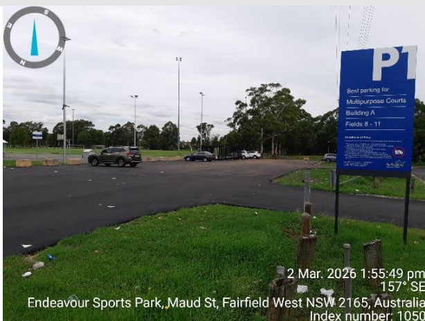
Car Park Renewal – MPCR2605 – Endeavour Sports Reserve near Baragoola Street Car Park. Rebuild the base and resurface with hot mix asphalt overlay
