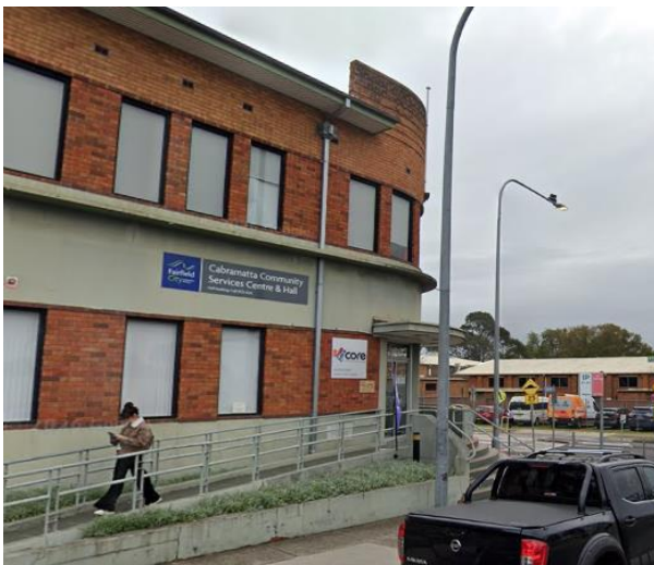
Figure 1 – Flaking and worn façade before works at the Cabramatta Community Centre.
