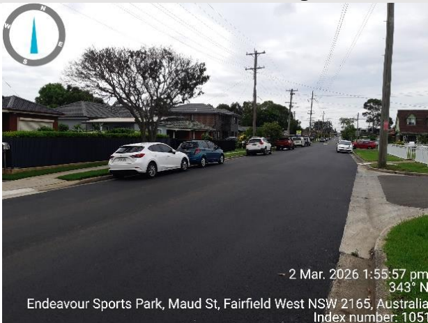
Resurfacing – MPRR2643 – Maud Street and Baragoola Street - from Thorney Road to Kambala Crescent
